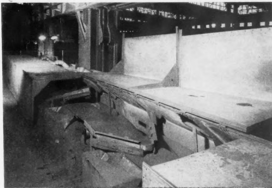
FIG. 7—Ventilated enclosure over sand plows above storage bin. Two hood sections have been opened for inspection. Note 4-in. slot along the floor level of enclosure. Photo courtesy Buffalo Forge Co.
